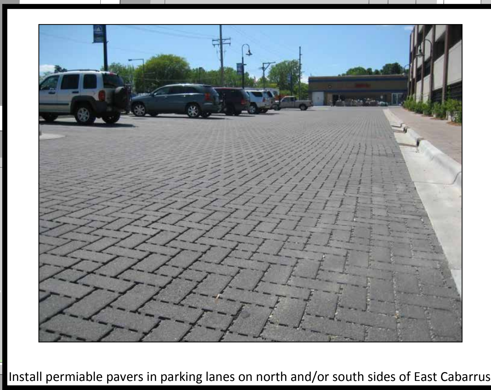
Install permeable pavers in parking lanes on north and/or south sides of East Cabarrus.
