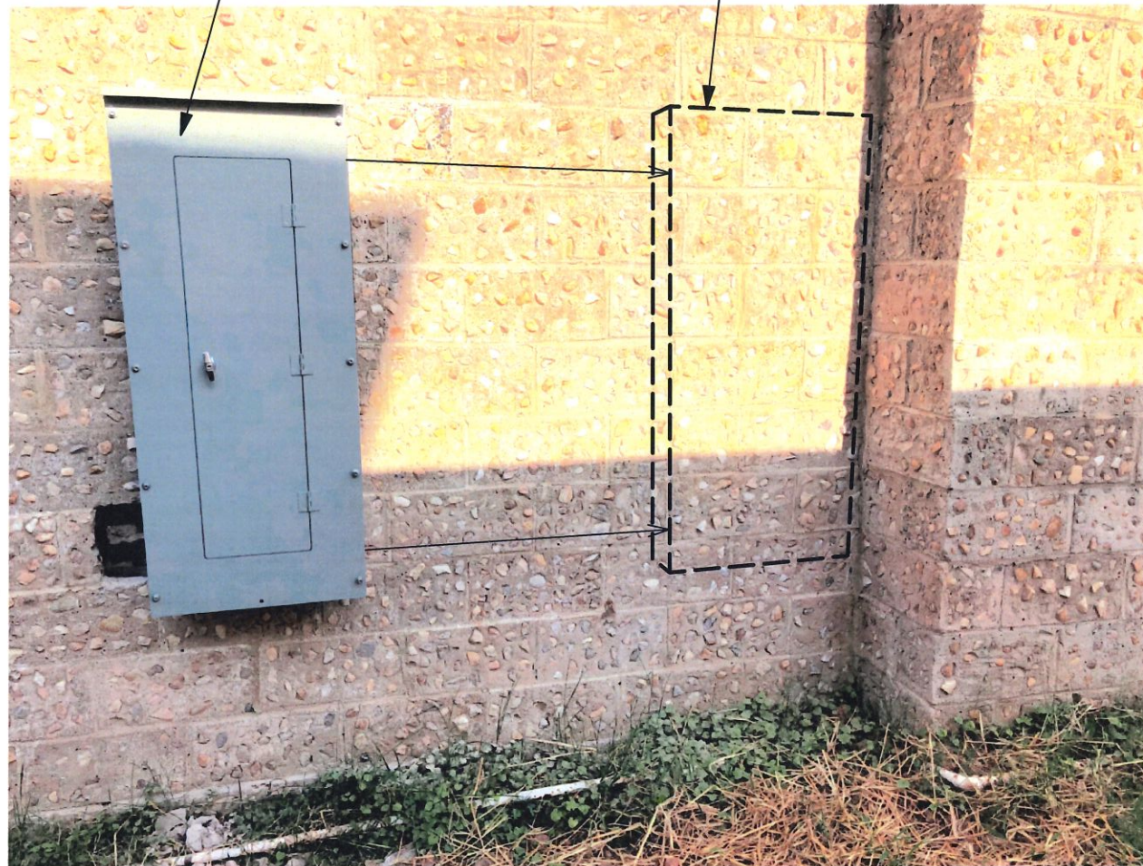
CURRENT PHOTO OF INSTALLED ELECTRICAL PANEL AT EAST FACADE
