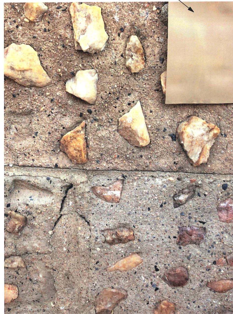
PHOTO OF PAINT CHIP AND EXISTING MASONRY/STONE. ELECTRICAL PANEL TO BE PAINTED TO MATCH MASONRY/STONE. EXISTING ADDITION SIDES TO BE PAINTED TO MATCH MASONRY/STONE.
