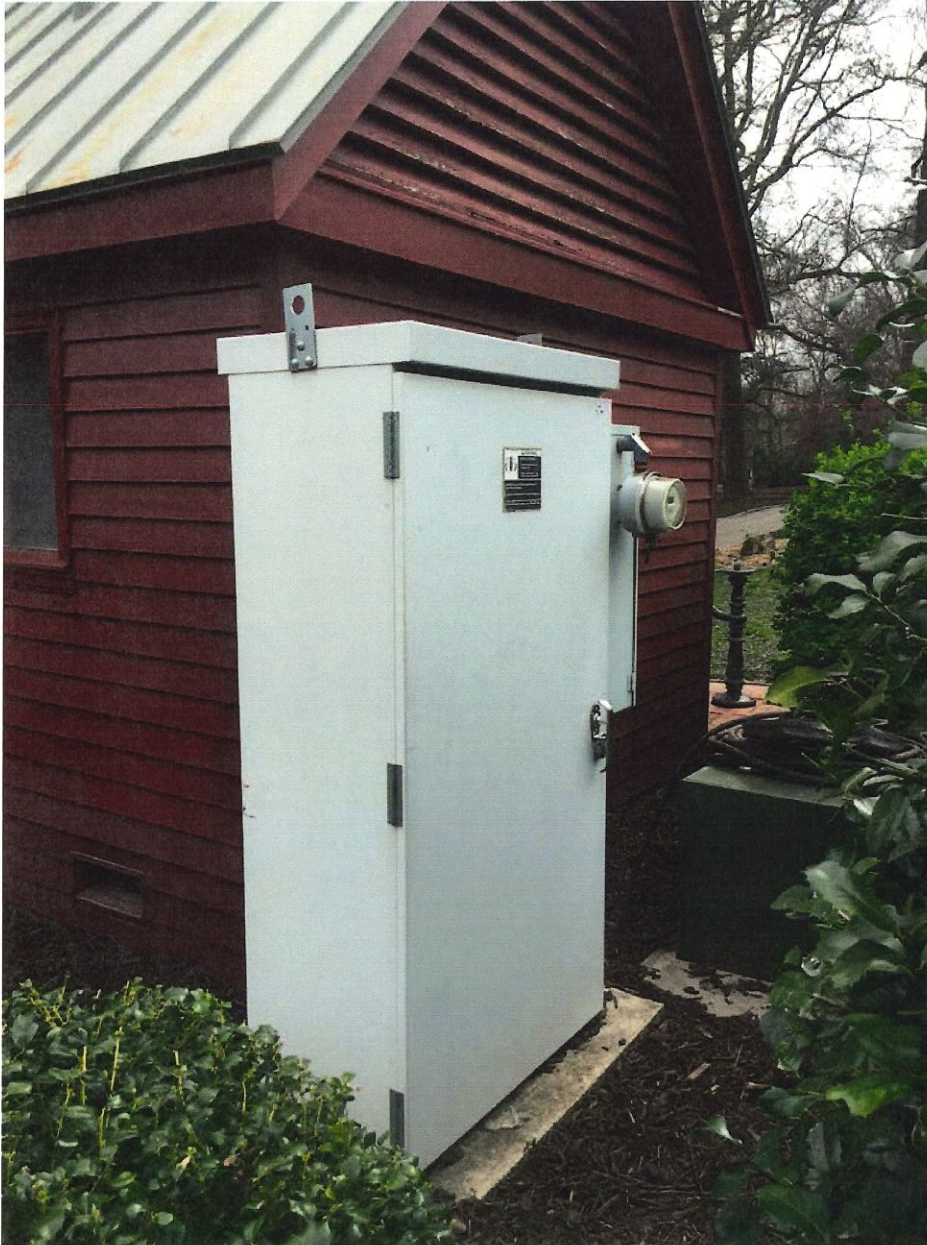
Similar Panel Installation-Currently on site adjacent to Restrooms Reference Sheet 2 CoA Application Photo Sheet - 3
