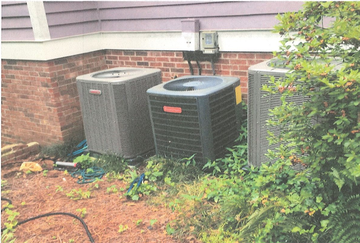
HVAC equipment in North side yard.
