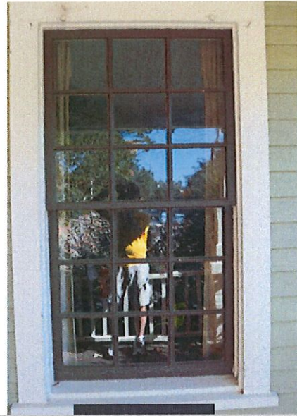
9 x 9 Double Hung Windows to be changed to 9 x 1 type per original design when home was constructed. All trim to remain the same.
