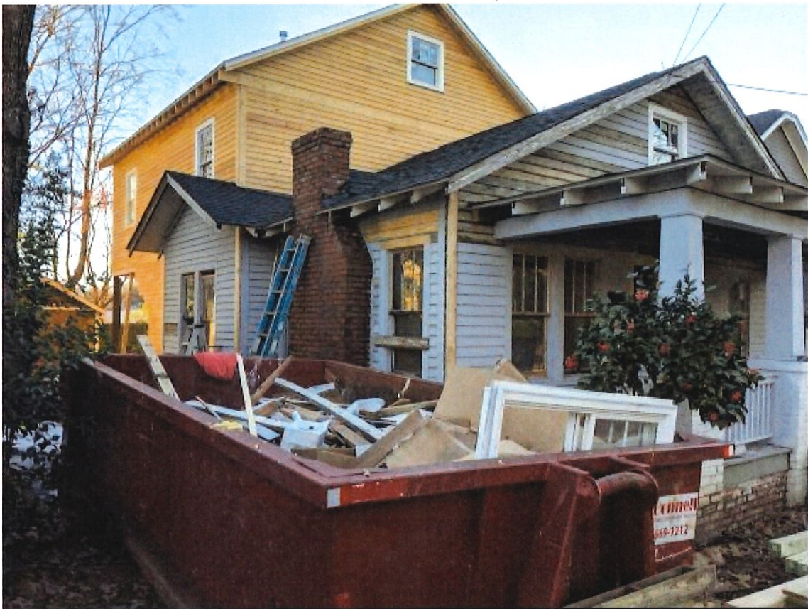
PHOTO#4 (current left side condition)
