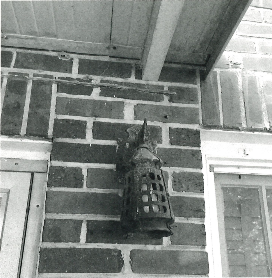
Photo G: Close-up of Evidence of Previous Awning at Front Door (Right Side)
