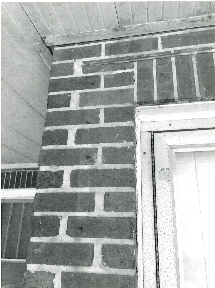
Photo F: Close-up of Evidence of Previous Awning at Front Door (Left Side)
