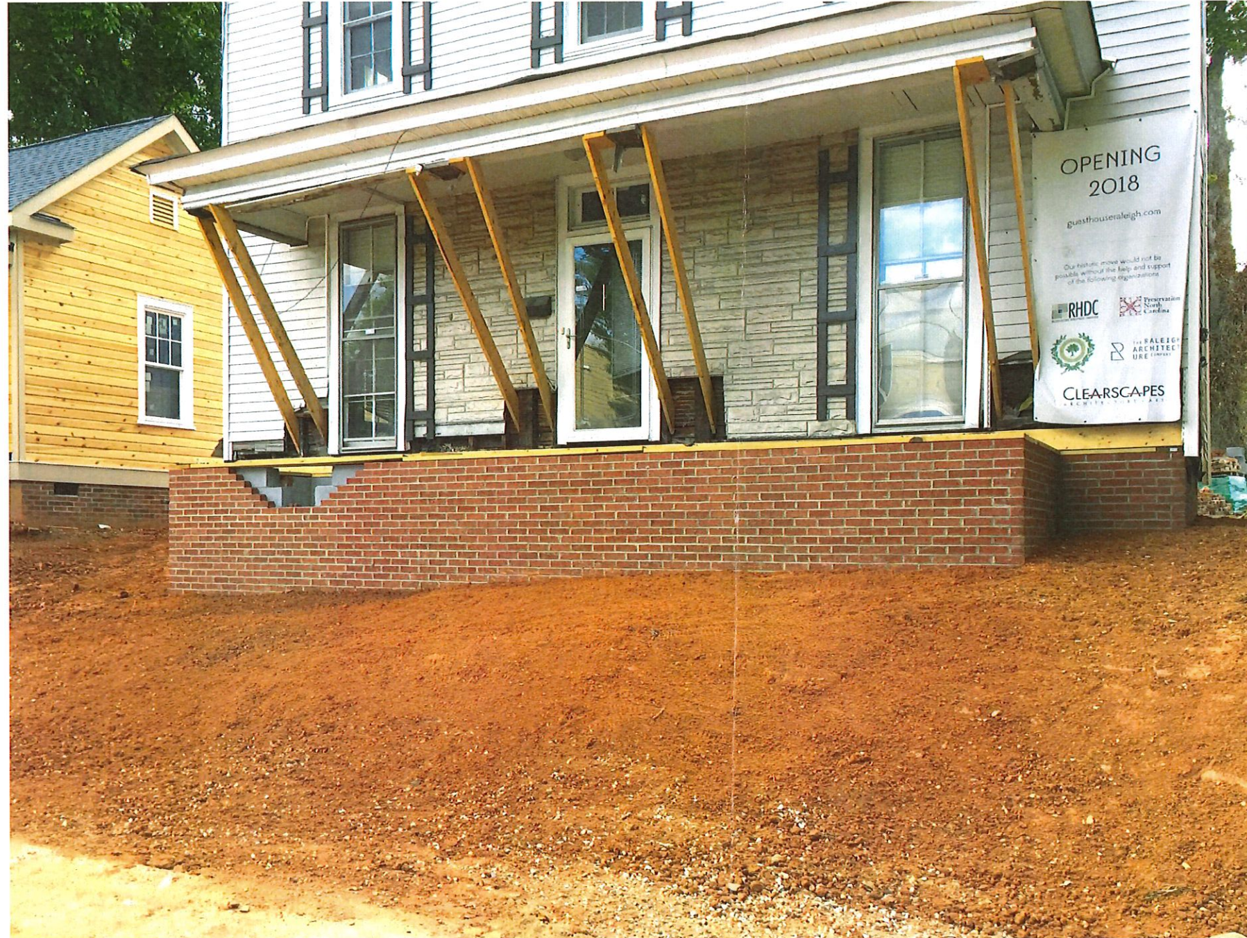
EXISTING PHOTO OF PROJECT SITE - FOUNDATION WALLS AND GRADING ALMOST COMPLETE AFTER HOUSE MOVE.
