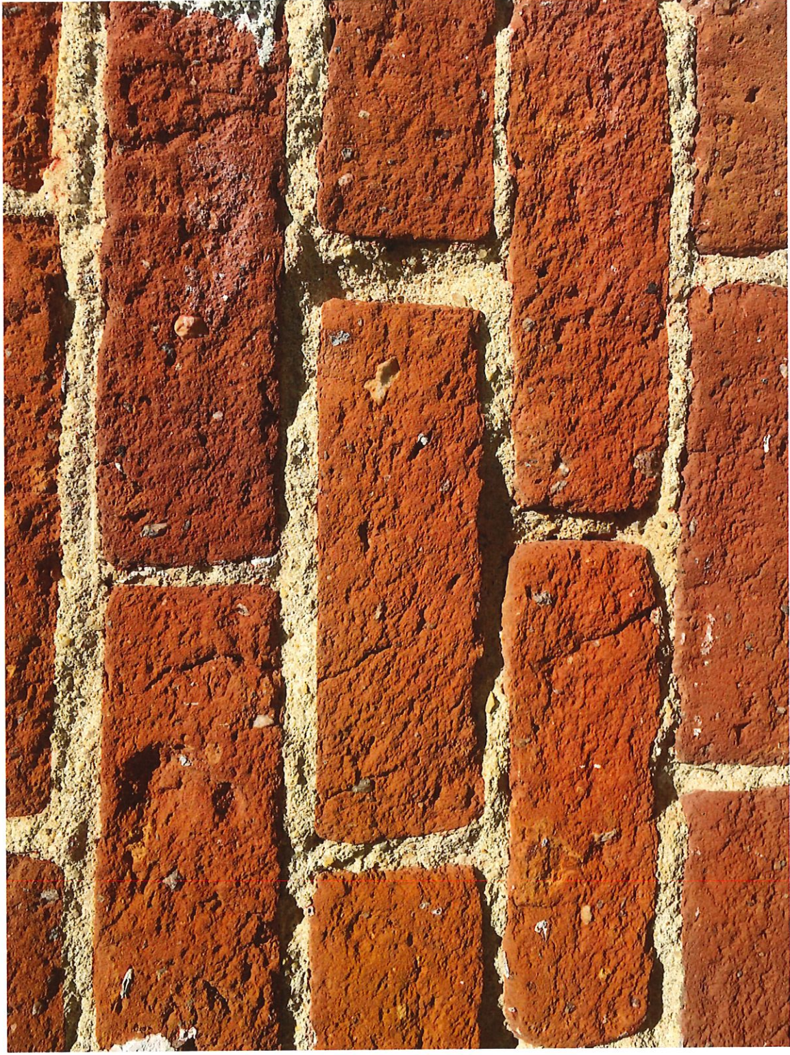
Existing brick at 519 Oakwood (note surface pitting from previous sandblasting) ADWSE
