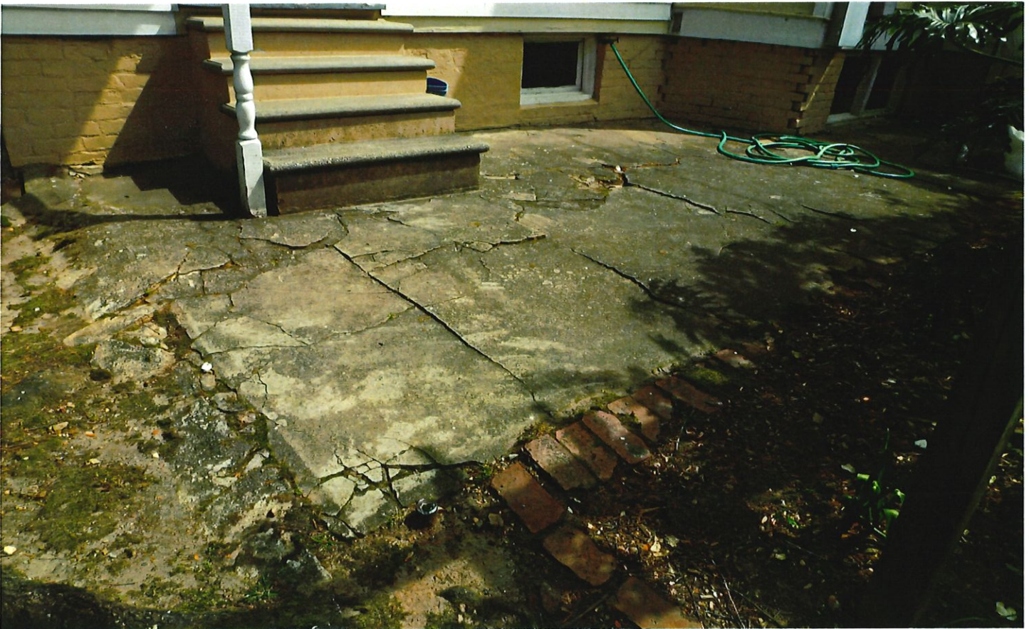
5 DETERIORATED CONCRETE PATIO W/ BRICK EDGE
