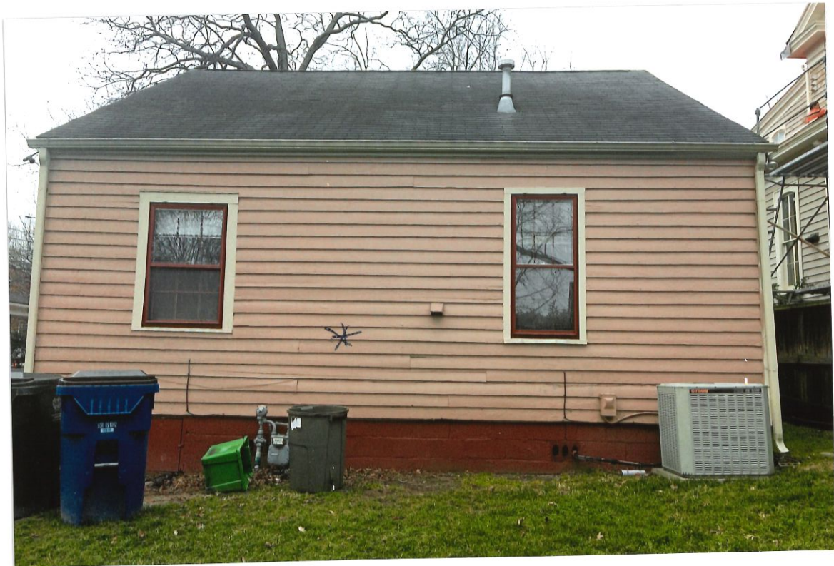
Back: Door Added to back to access deck Deck added to back of house owner: Loureen Hall
