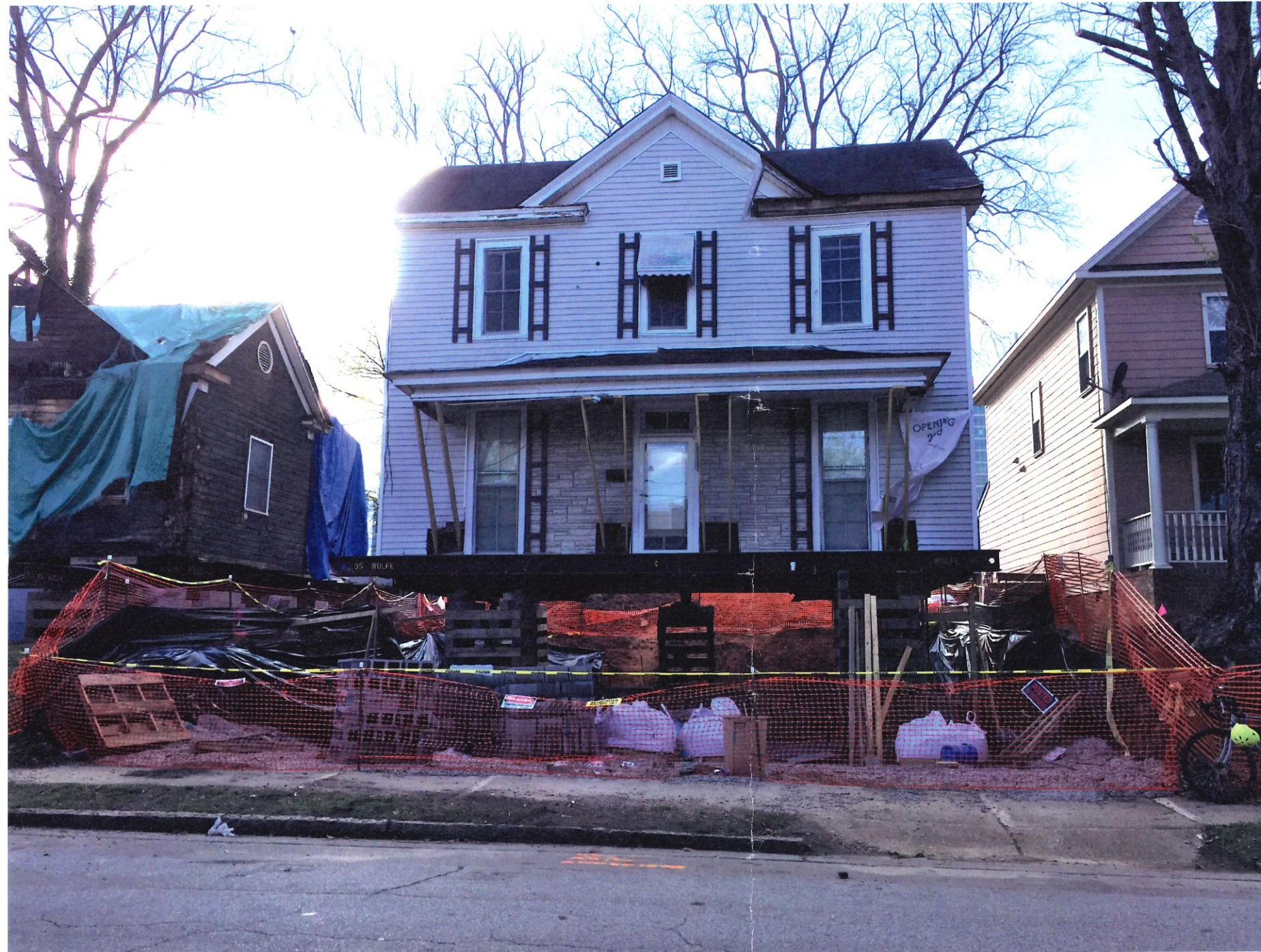
EXISTING PHOTO OF PROJECT SITE - FOUNDATION WALLS CURRENTLY UNDER CONSTRUCTION AFTER HOUSE MOVE.
