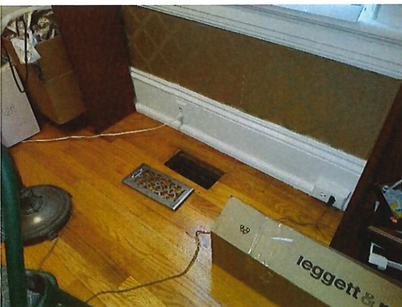
Picture 5 – Hump in floor at front room
