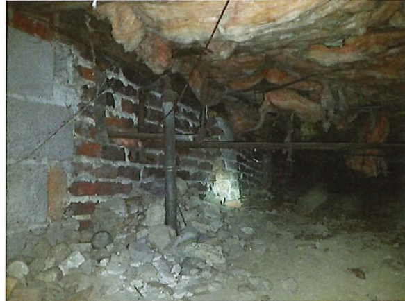
Picture 2 – Example of leaning pier/curtain wall
