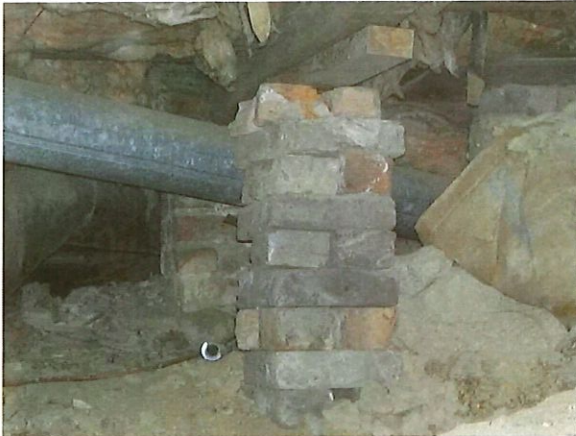
Picture 7 – Deteriorated masonry piers along leftmost girder
