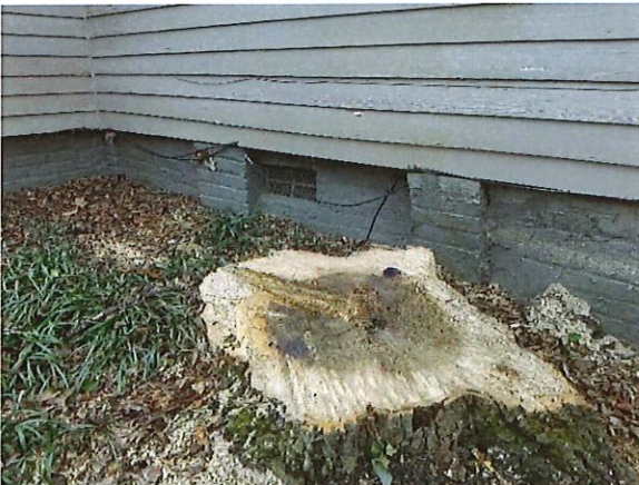
Picture 3 – Example of leaning pier/curtain wall
