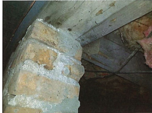
Picture 8 – Inadequate support at front end of leftmost girder
