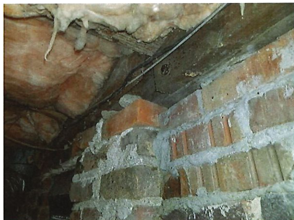
Picture 6 – Damaged perimeter rim beam
