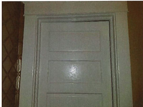
Picture 4 – Racked interior doorway at front room
