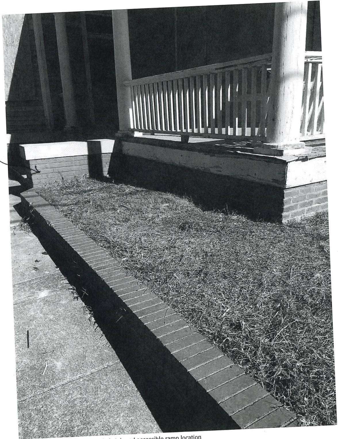
image of existing brick at modified stair and accessible ramp location 219 E North Street Certificate of Appropriateness from Raleigh Historic Districts Commission
