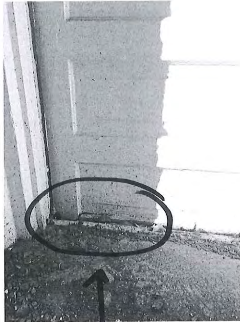
Door #1 Rotting/ Damage Exterior
