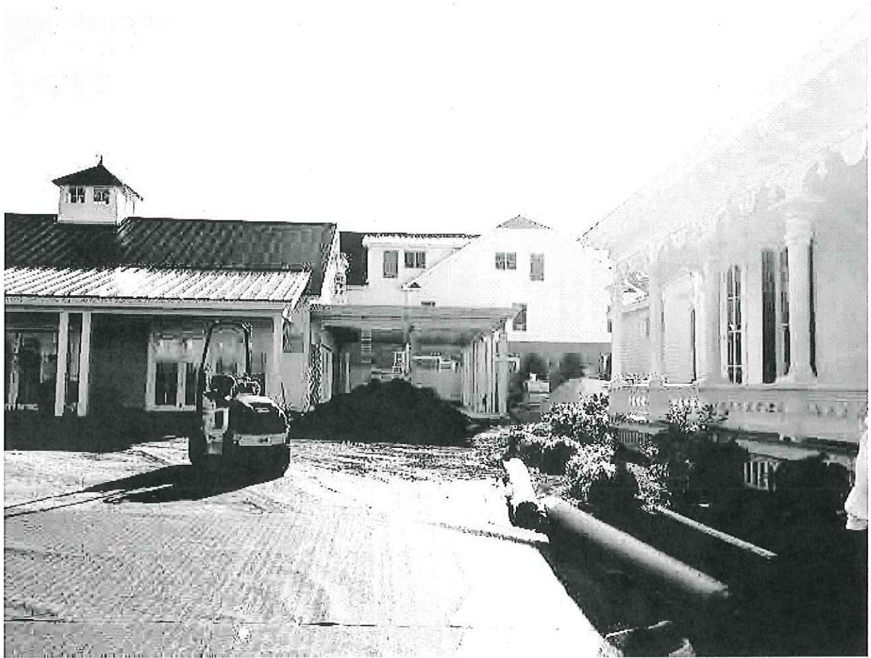
View from the west of the structure with side of The Merrimiion-Wynne house
