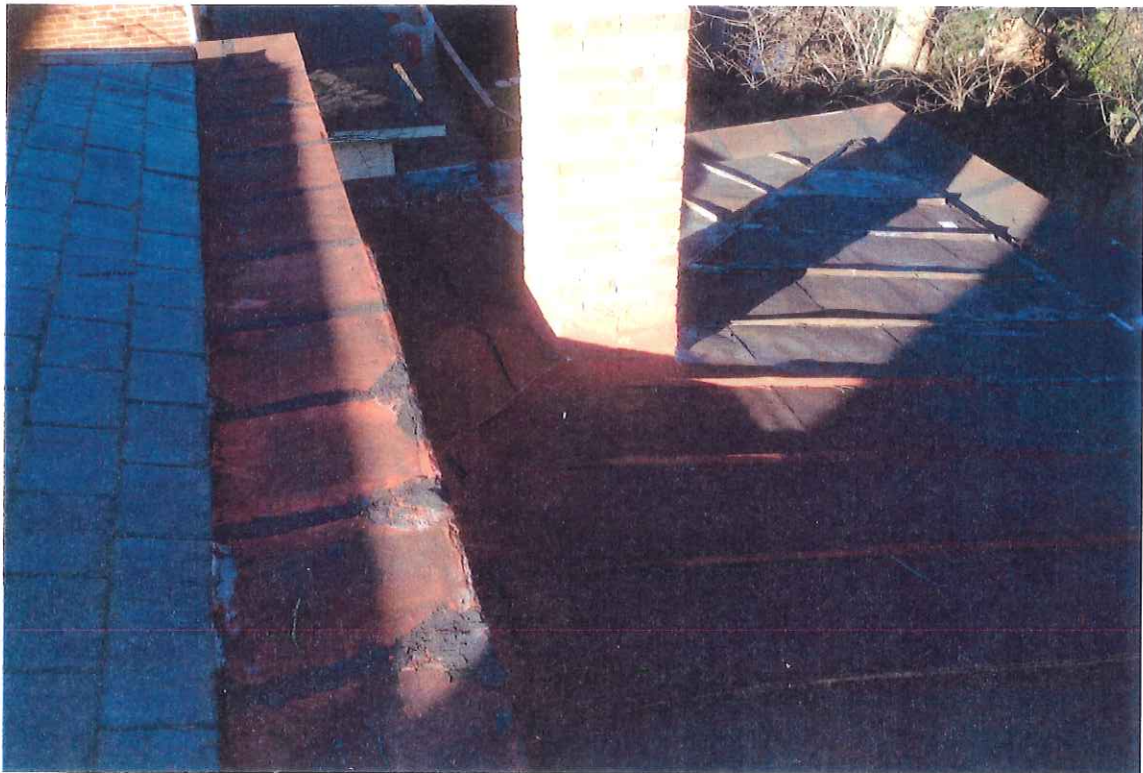
same as above, showing non-functioning chimney that I request to remove in this minor work COA application
