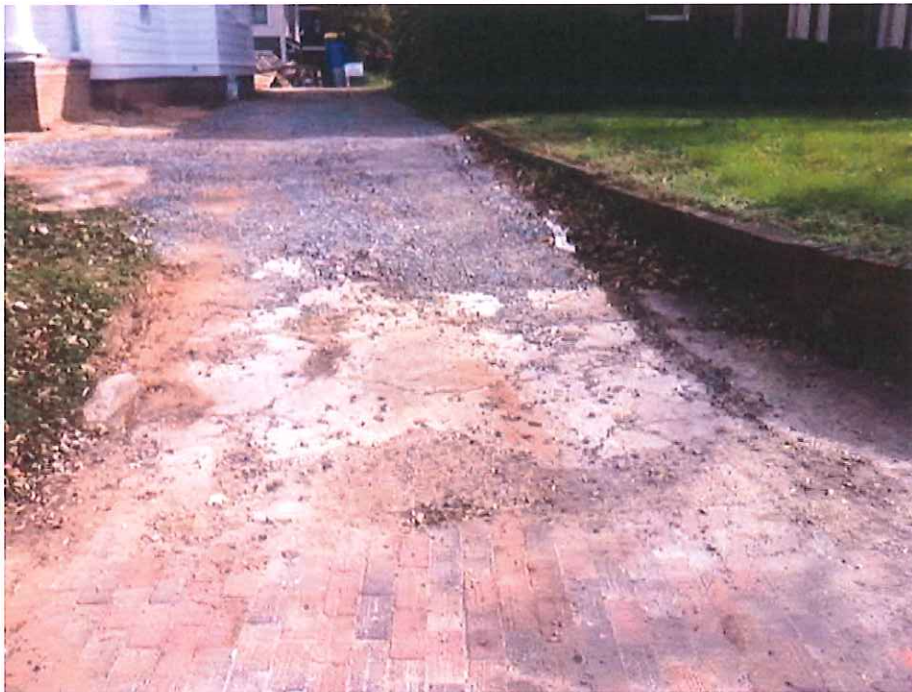
Photo 3,4,5: Shows the current damage to the concrete entrance to the driveway.
