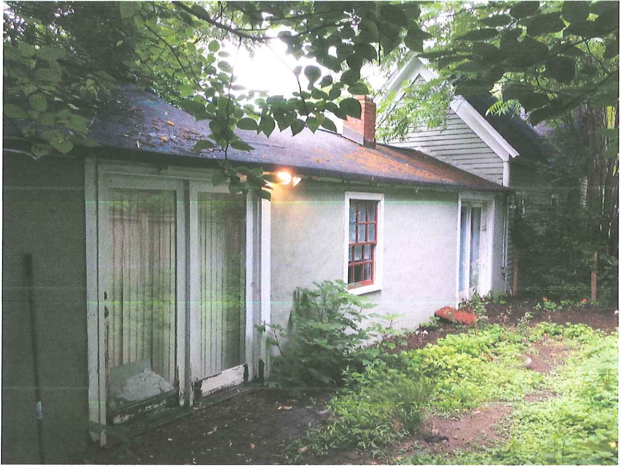
Rear addition, patio doors that will be changed + masonry flue that will be removed
