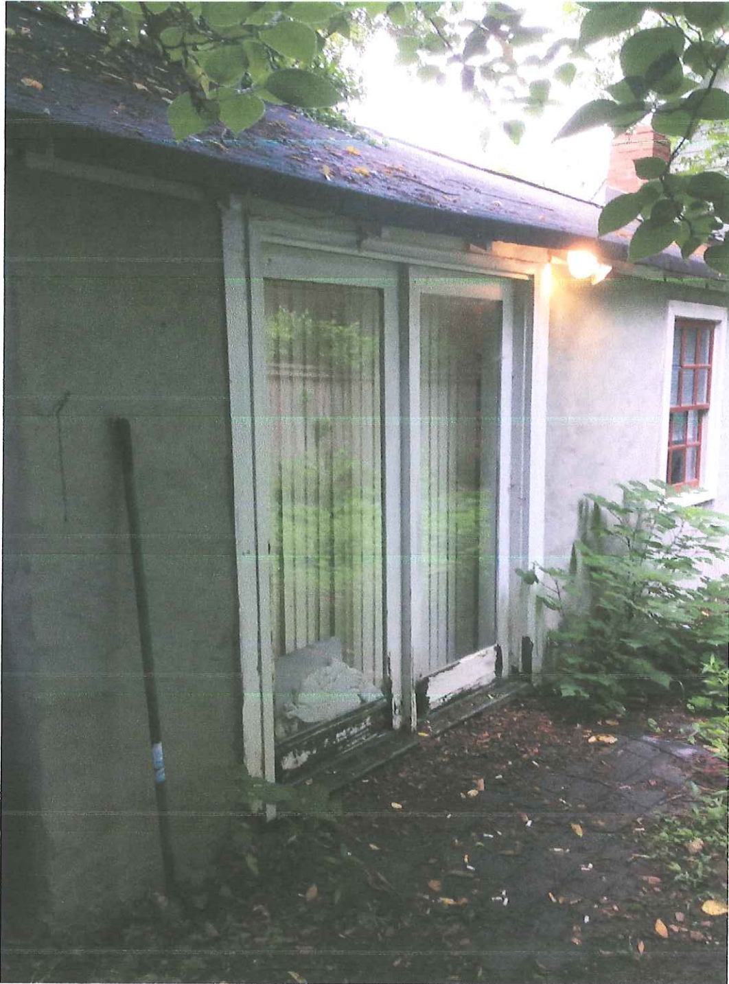
Existing wood full lite pair of doors that owners would like to change to a pair of wood windows (ganged) that fit into the same rough opening as the patio doors. Sill will be raised with a low cmu wall, parged and painted to match existing exterior wall.
