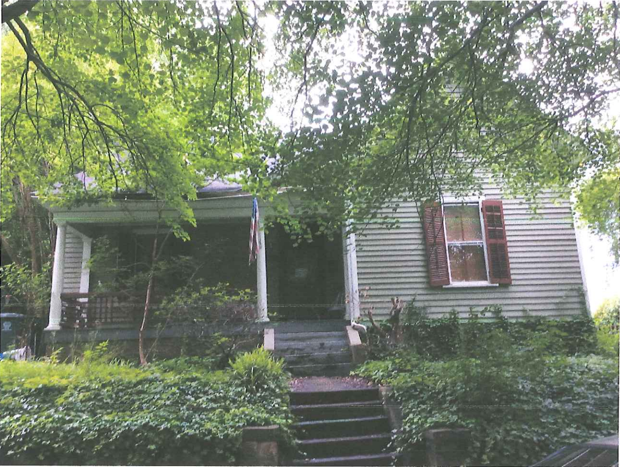
Front Elevation of 223 Elm St – Gutter damage is seen on front porch
