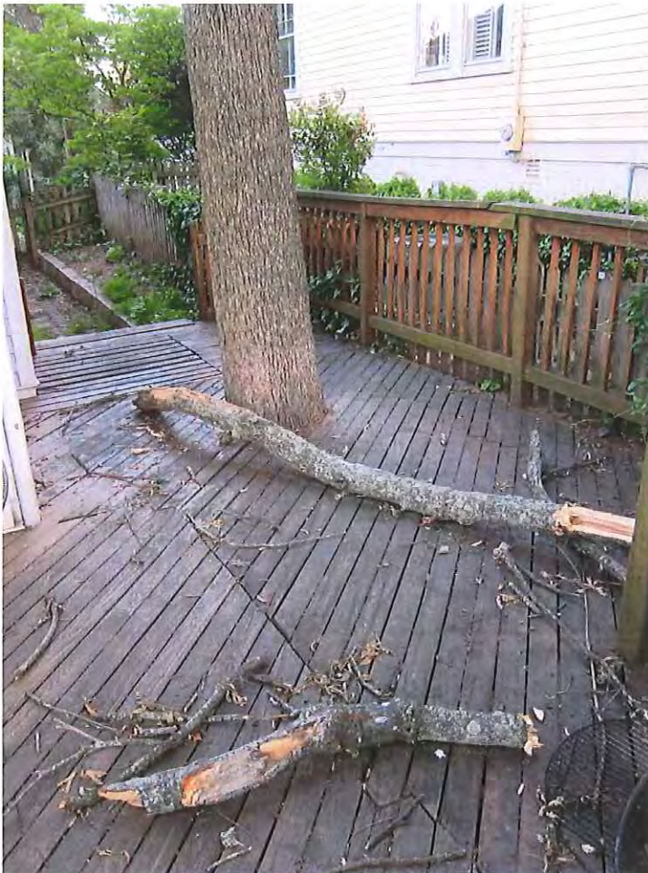
Figure 8: Taken from deck showing limb which recently fell during a storm and potential hazard of tree.
