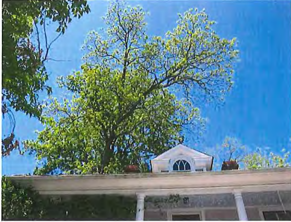
Figure 3: Taken from front of house showing how far over the house the tree extends.
