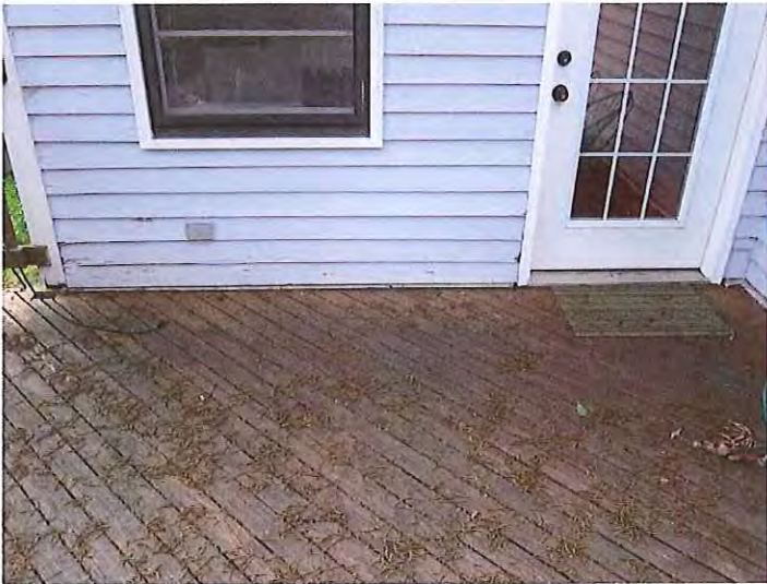
Figure 10: Edge of deck touching back section of house
