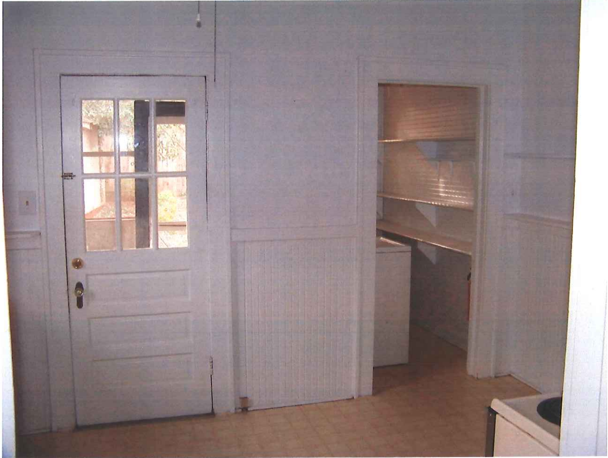
Existing rear entry door to be reinstalled at newly enclosed screen porch
