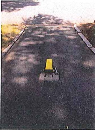
Existing bollard (broken) west entrance from Mordecai Drive
