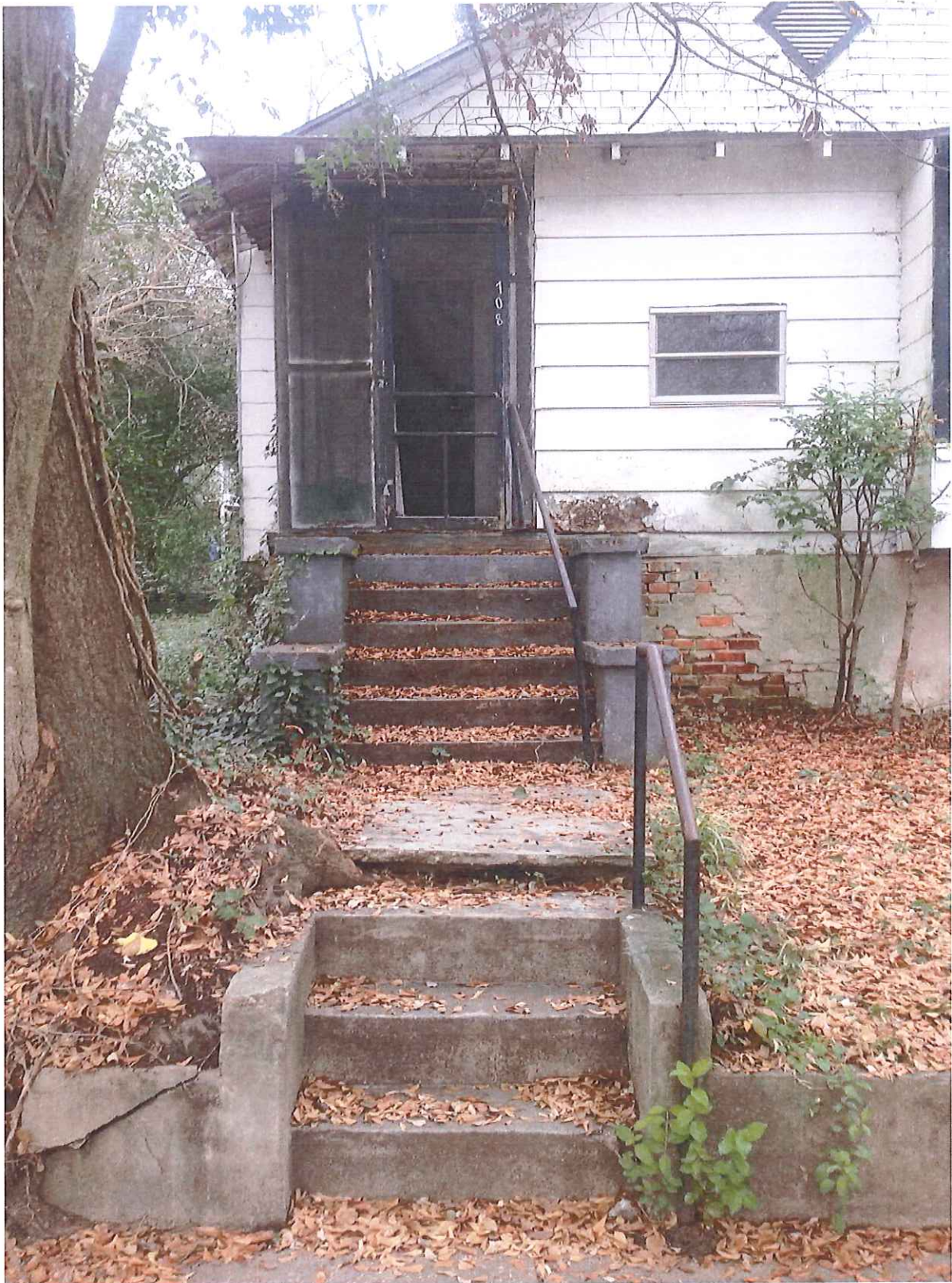
Figure 2 Damaged steps and concrete walkway to be replaced in kind
