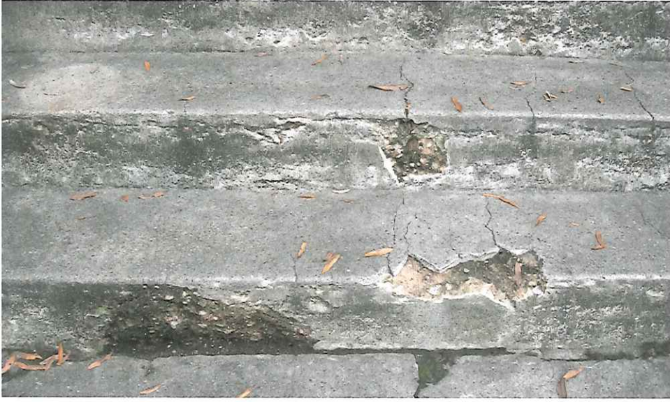
EXISTING LOWER 2 STEPS / DETEIORATED
