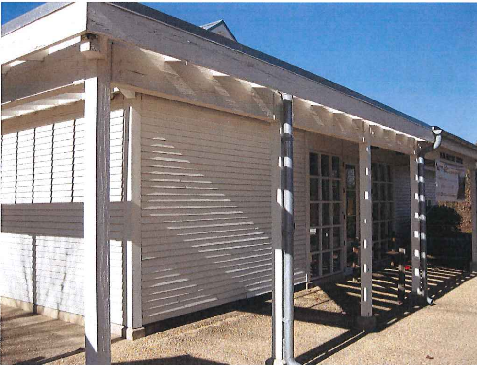
FARM HISTORY MUSEUM - CORNER TO BE REPAIRED
