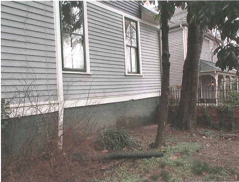
Figure 1: proposed location of AC units, under the windows, between the foundation and trees
