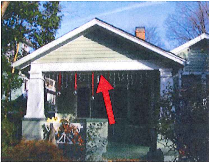
Front view of house showing porch. Arrow shows approximate location for proposed fan.
