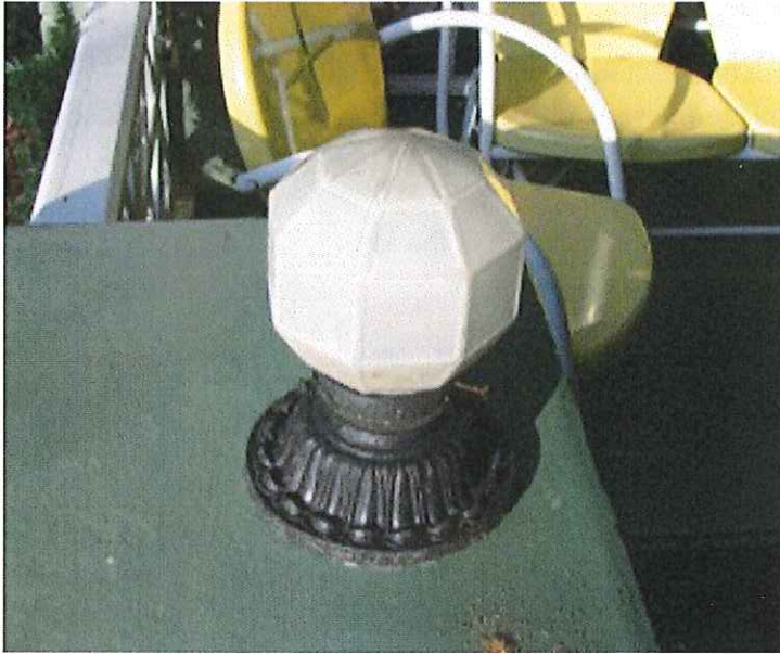
Existing fixture to be replaced.
