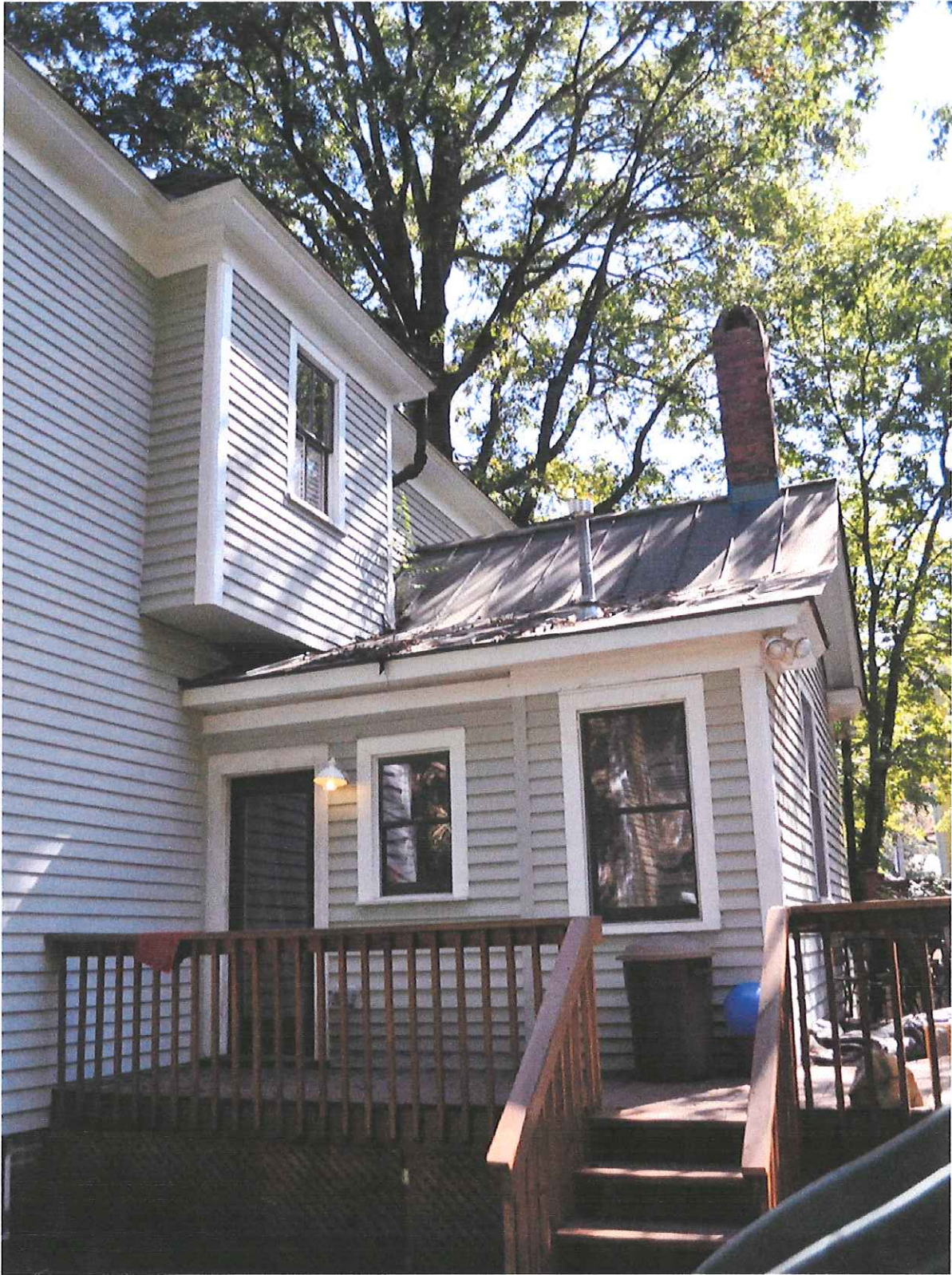
Existing Elevation of Mudroom + Laundry Room - door to be removed and small window to be replaced by a larger window to match laundry room window. More consistent appearance
