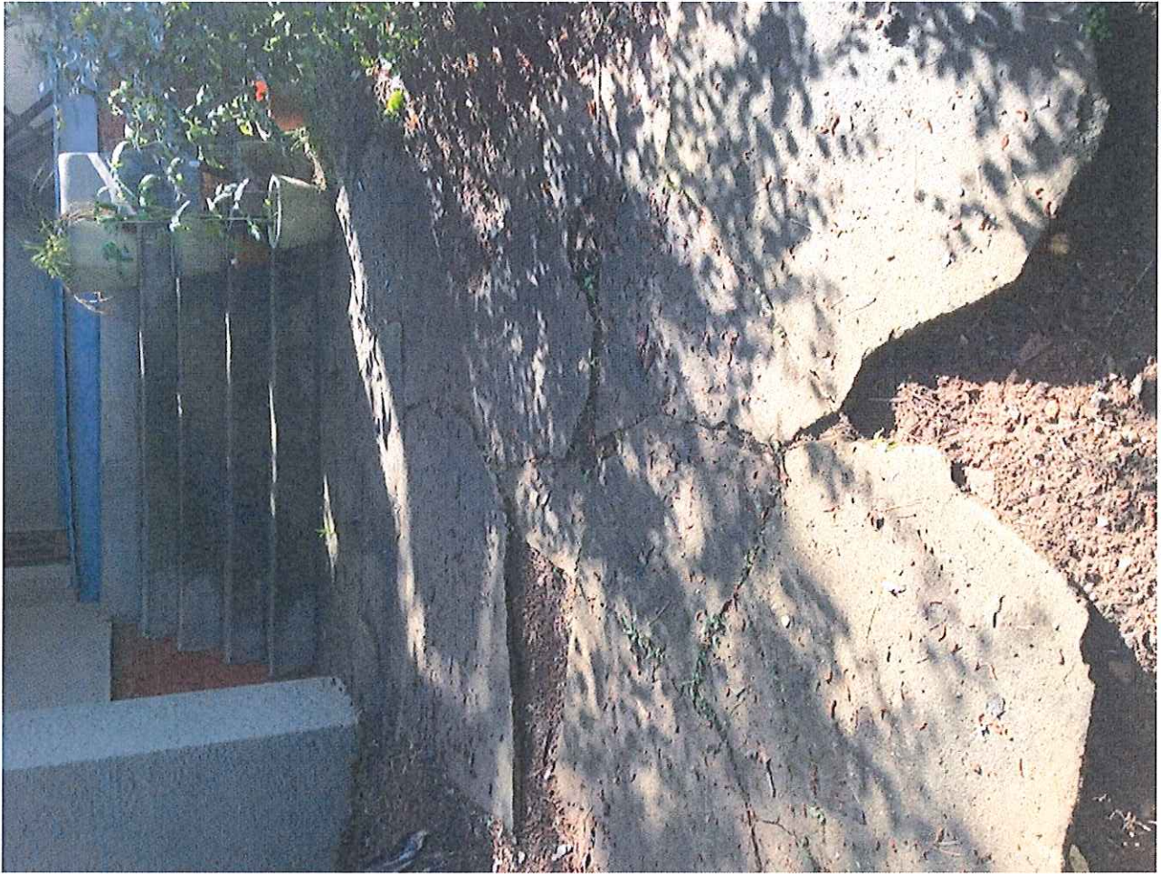
Broken Front Walkway
