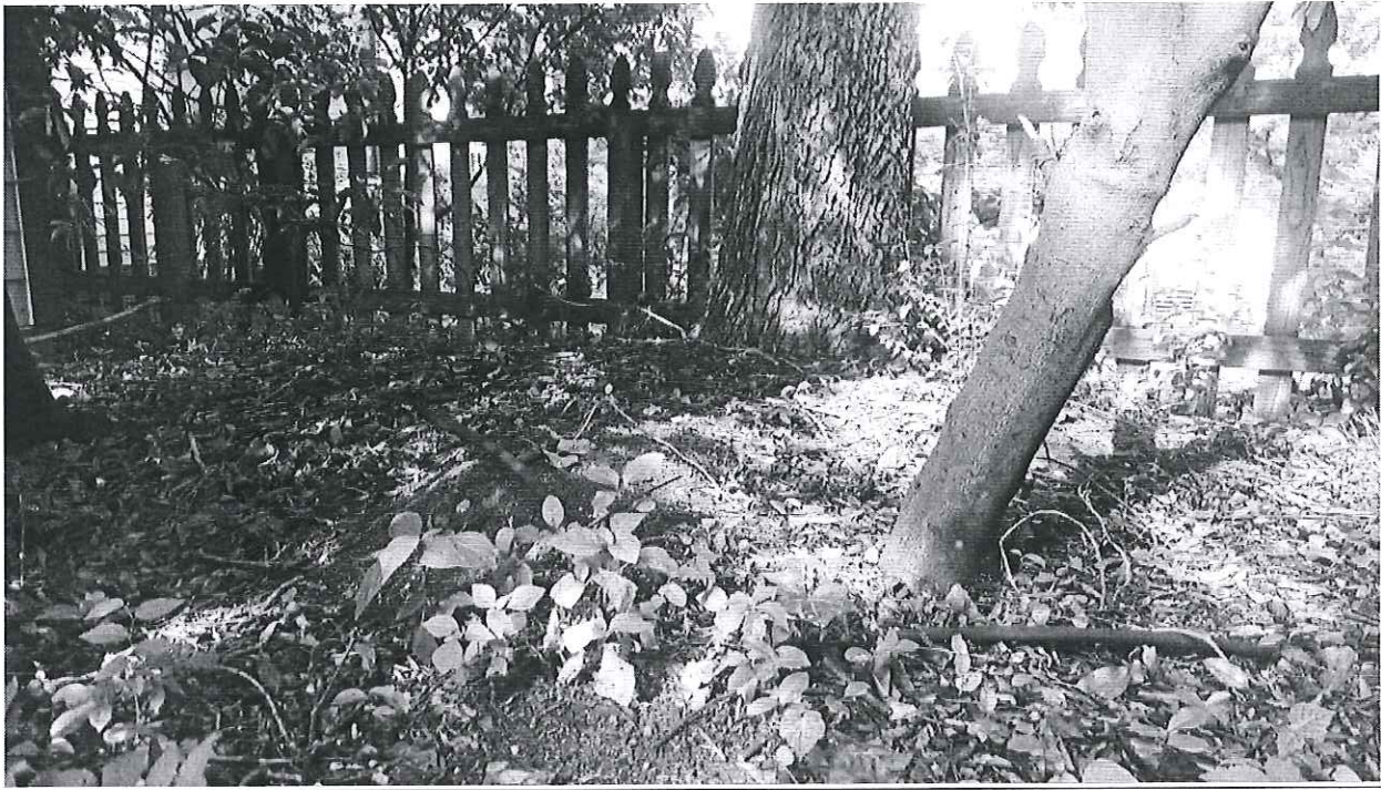
Photo 2 – Roots of tree bulging from ground
