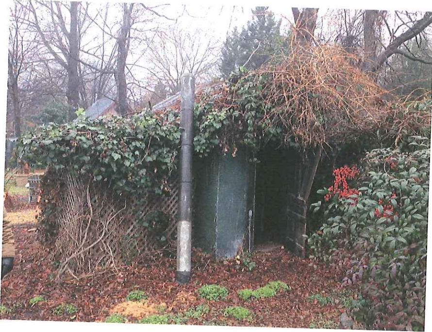
View of existing shed at 403 Elm. This structure has a dirt floor and rotting wood walls. It is unsafe for use in its current condition, and is being completely overgrown by weeds and unkept ground cover.
